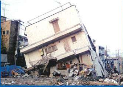
1 階片側の柱が折れ、大きく傾いた3階建ての住宅 神戸市東灘区 1995.2.26 A broken support pillar on one side of the ground floor caused this three storey house to tilt severely. Higashi Nada Ward, Kobe City. 26 February 1995.
