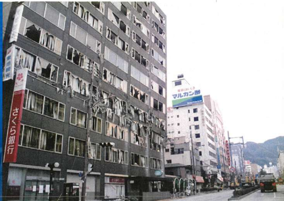
神戸の中心部、三宮の破損したビル。よく見ると4階部分がつぶれ、3階の上に5階部分が乗った状態に 神戸市中央区 1995.1.21 Damaged building in Sannomiya, central Kobe. The fourth floor has completely collapsed and the fifth floor now sits on top of the third floor. Chuo Ward, Kobe City. 21 January 1995.
