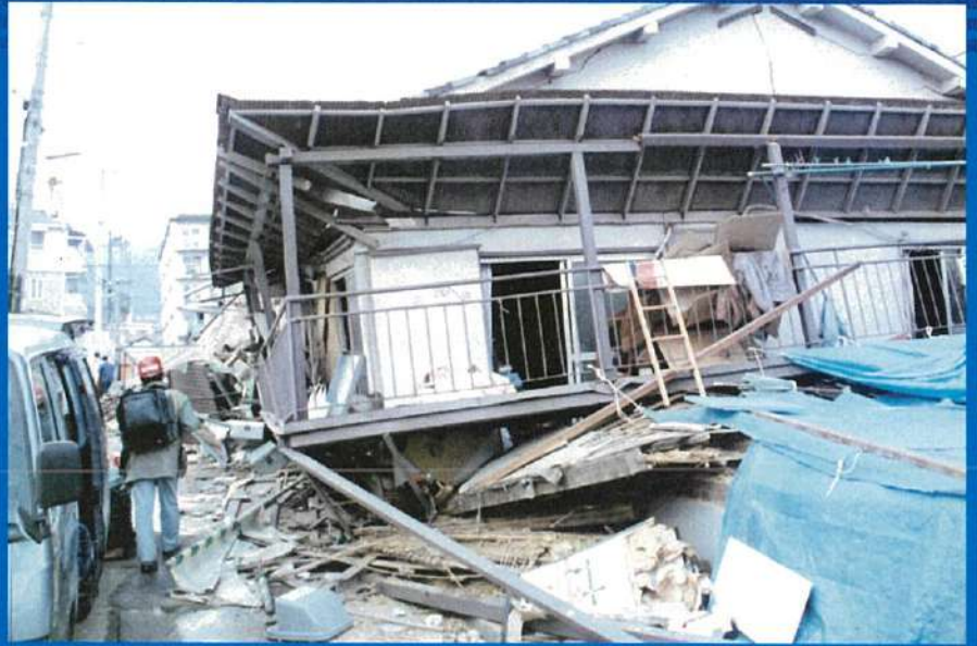
1階部分がつぶれ2階が地上まで倒壊した住宅 神戸市灘区 1995.1.21 The ground floor of this house collapsed, and the second floor has come to the ground. Nada Ward, Kobe City. 21 January 1995.
