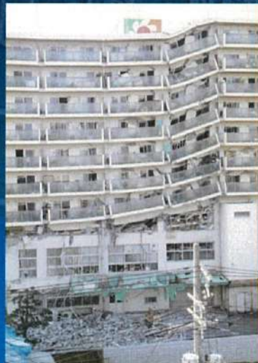
高層住宅の被災。低層の特定の階だけがつぶれ歪みが生じている 西宮市 1995.2.26 Damaged high rise apartment block. Lower level floors have collapsed, distorting the building structure. Minatogami City. 26 February 1995.
