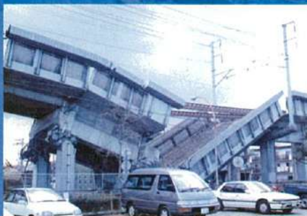
鉄道の高架線路の一部が外れて地上に落ちている 西宮市 1995.1.24 Part of an elevated railway has broken away and falls. Nishinomiya City. 24 January 1995.
