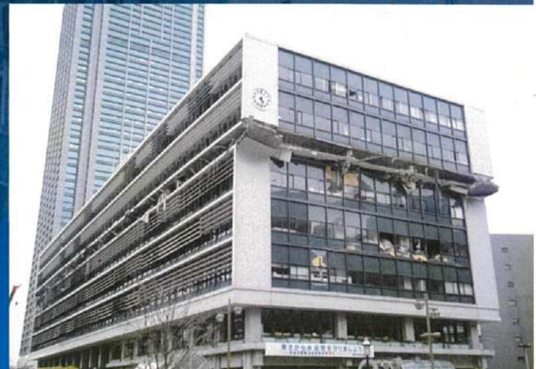
8階建ての6階部分がつぶれた神戸市庁舎2号館。その後、6階より上層を除去し5階建ての建物として再建された 神戸市中央区 1995.1.23 Kobe City No. 2 government office building. The sixth floor of the eight storey building has collapsed. It has been reconstructed as a five storey building, with the upper floors removed. Chuo Ward, Kobe City. 23 January 1995.
